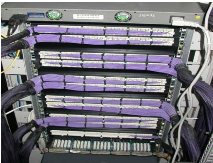
LSZH Cat 5e cable and multi core telecom cable installed into the rear of a comms cabinet
