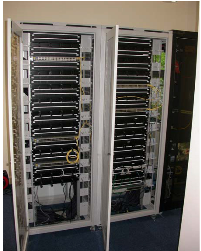
Two of the comms cabinets (front view) before patching
